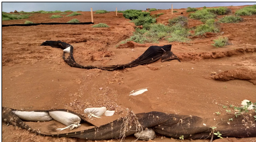
Figure 38 Check dams installed in 2015 and damaged by a large storm event
