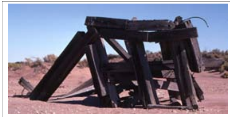
Figure 6 Two views of jetty remnant; one showing location to dune system
