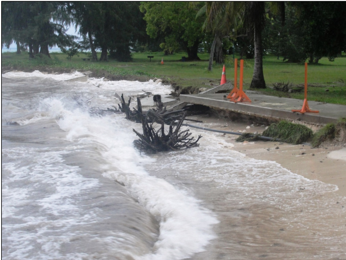
Figure 26. A section of collapsed sidewalk and adjacent eroded shoreline during a high tide and large west swell at American Memorial Park (Photo by R. Greene 2013).
