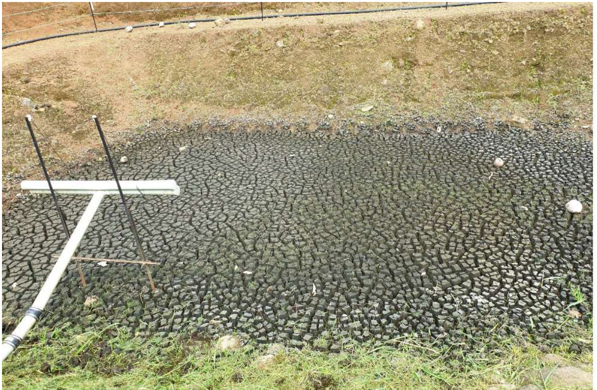
Figure 15 – Ngatoe scour pond (12 Jan 2021)
