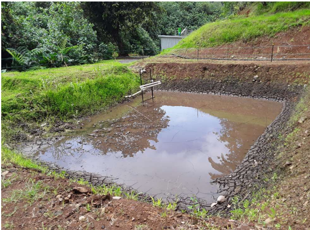
Figure 14 – Ngatoe scour pond after a heavy rain (12 Dec 2020)
