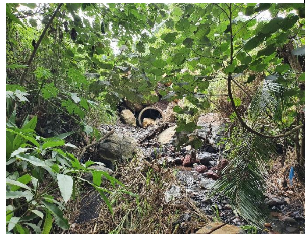
Photograph 4.4: Culvert along Vairauara Stream, some shallow pools of water present in foreground, May 2021.
