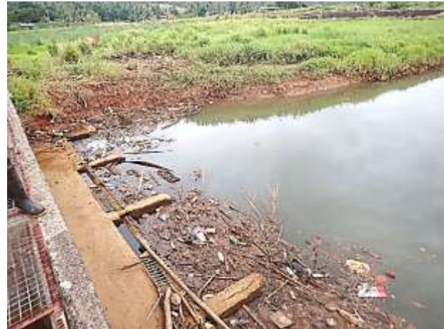
d) Rubbish clogging the floodgate
