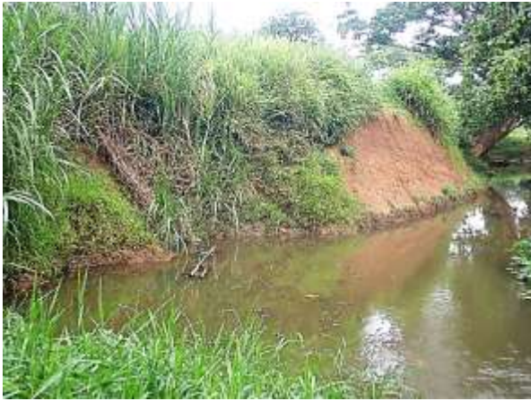
c) FW4: Eroded bank, highly modified riparian zone, silted streambed
